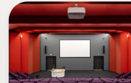
Ulster University Standardised AV systems for a more sustainable, connected, and flexible campus
